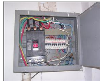
Photo of the inside of the main production hall NC-no internal safety cover for the power box.jpg
