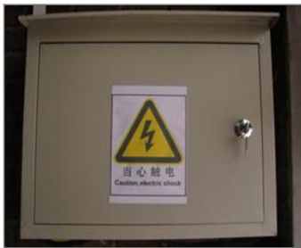
Photo of the inside of the main production hall Electric Box With Warning Sign.JPG
