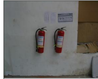
Photo of the inside of the main production hall Fire extinguishers 3.JPG
